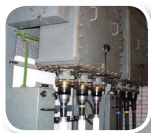
Power Sensitive Equipment
